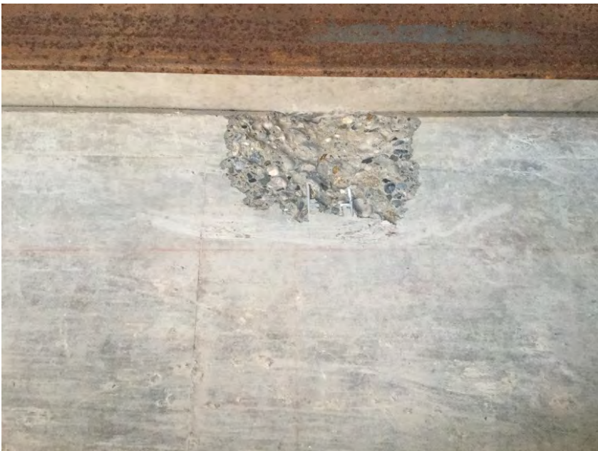
Small spall at left ballast wall
